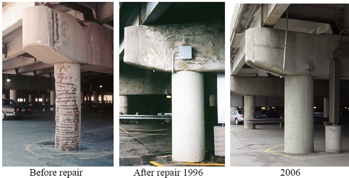
Figure 20: GFRP jacketed columns before and after repair [1]. Adapted with permission from Ref. [1]. Copyright ©2007.
