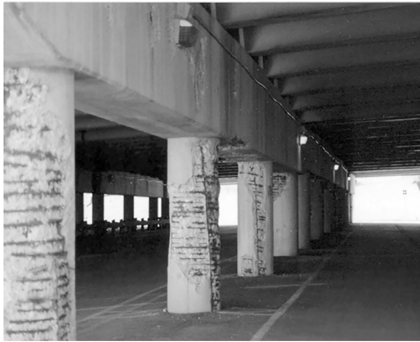
Figure 19: Damaged highway bridge columns [1]. Adapted with permission from Ref. [1]. Copyright ©2007.
