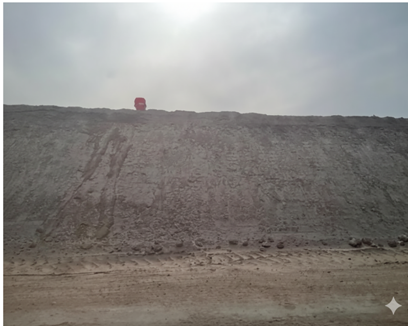
(b) Slope erosion (Location: k233+965.8)
