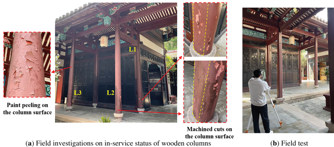
Figure 3: Field measurement of a traditional timber ancestral hall of Qing Dynasty in China.
