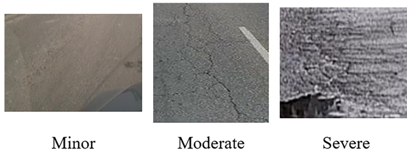
Figure 9: Three levels of road damage severity.
